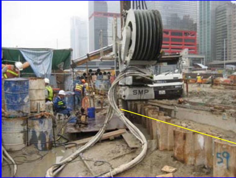
Alignment out-of-line when encountering obstructions
