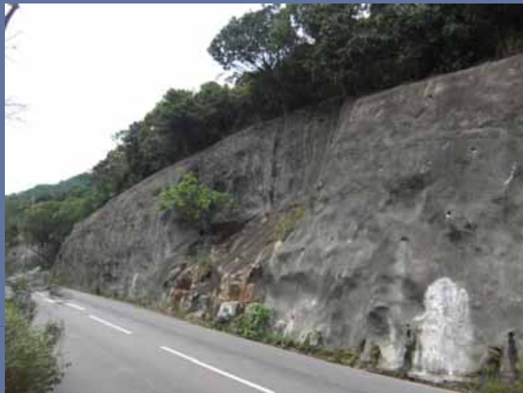
Planar Failure – Tai Tam Road
