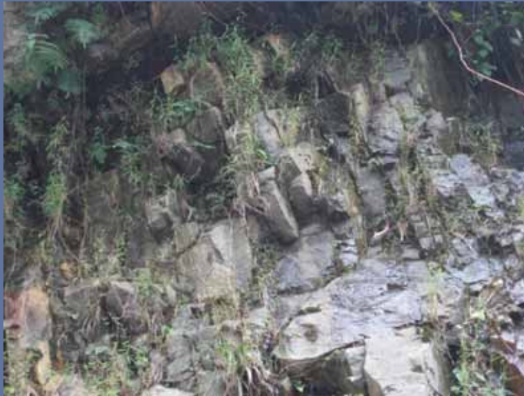
Ravelling Failure – Kennedy Road
