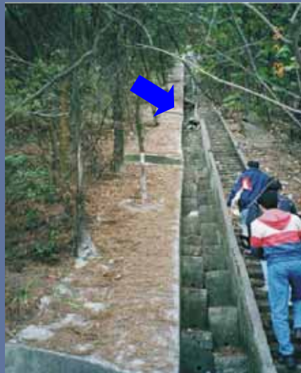
Collapse of side wall of surface channel
