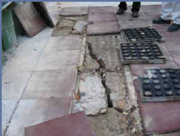
Tension crack at crest
