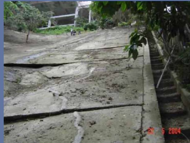
Subsidence of slope cover
