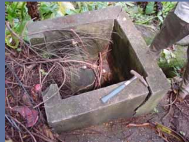
Cracking of catchpit
