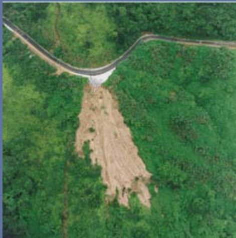
Au Tau Village Road Failure in 1998
