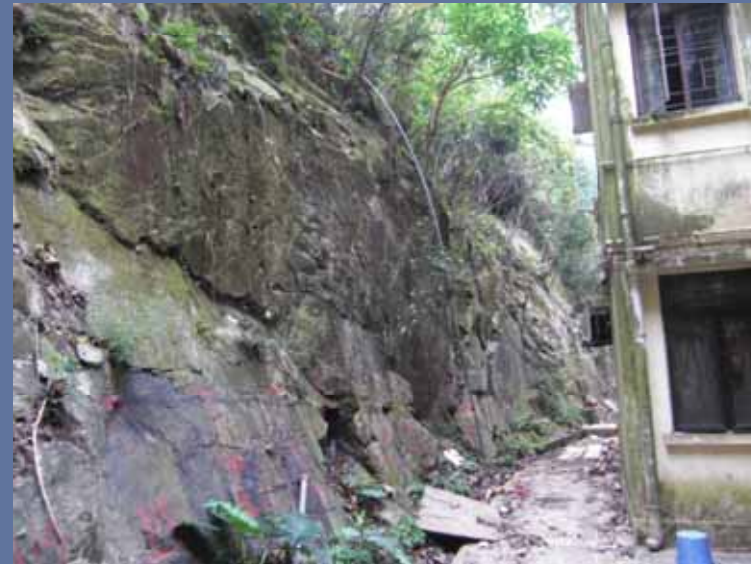
Wedge Failure – Pokfulam Road
