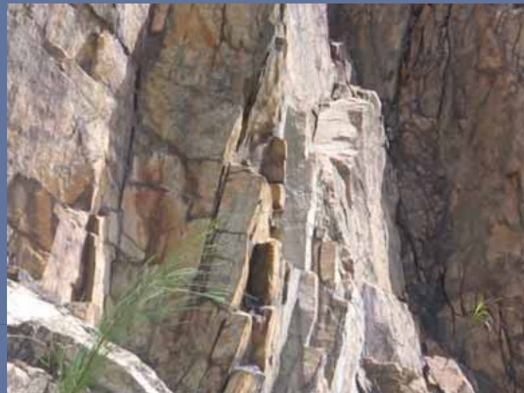
Toppling Failure – Mt Butler
