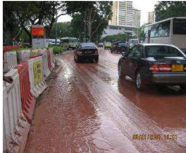
Loss of slurry onto road
