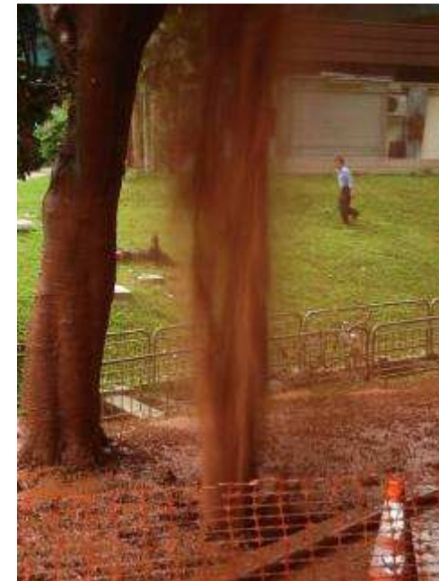
Leakage of air into the excavation chamber led to an 'airlift' effect up an old borehole
