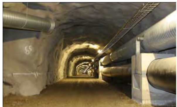
Fig. 9 Typical Utility Tunnel (Photo: Jorma Vilkmán)
