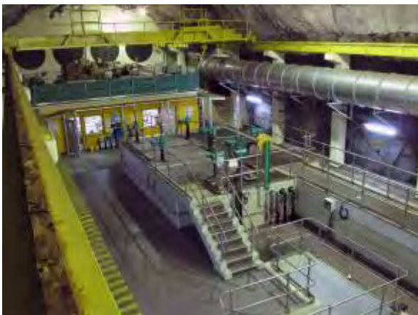
Fig. 10 Use of Overhead Crane in Service Area
