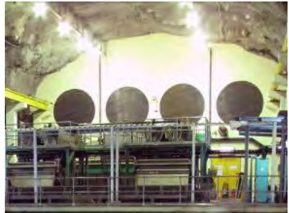
Fig. 7 Fresh Air Inlets
