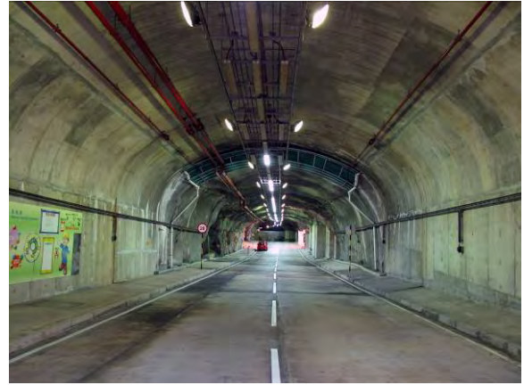
Fig. 11 Sprinkler System at Entrance Portal
