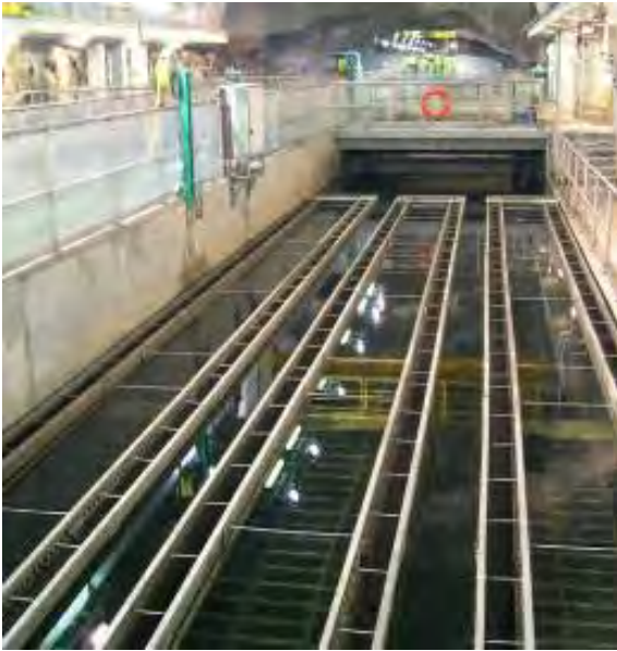
Fig. 5 Lamella Settlers in Final Sedimentation Tank
