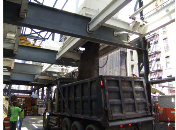
Fig. 8 Custom-designed Muck Handling System
