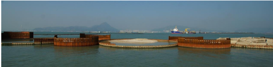
Figure 8. The cellular structure and arc units are completed and filled up with fill materials and the reclamation fill behind in progress
