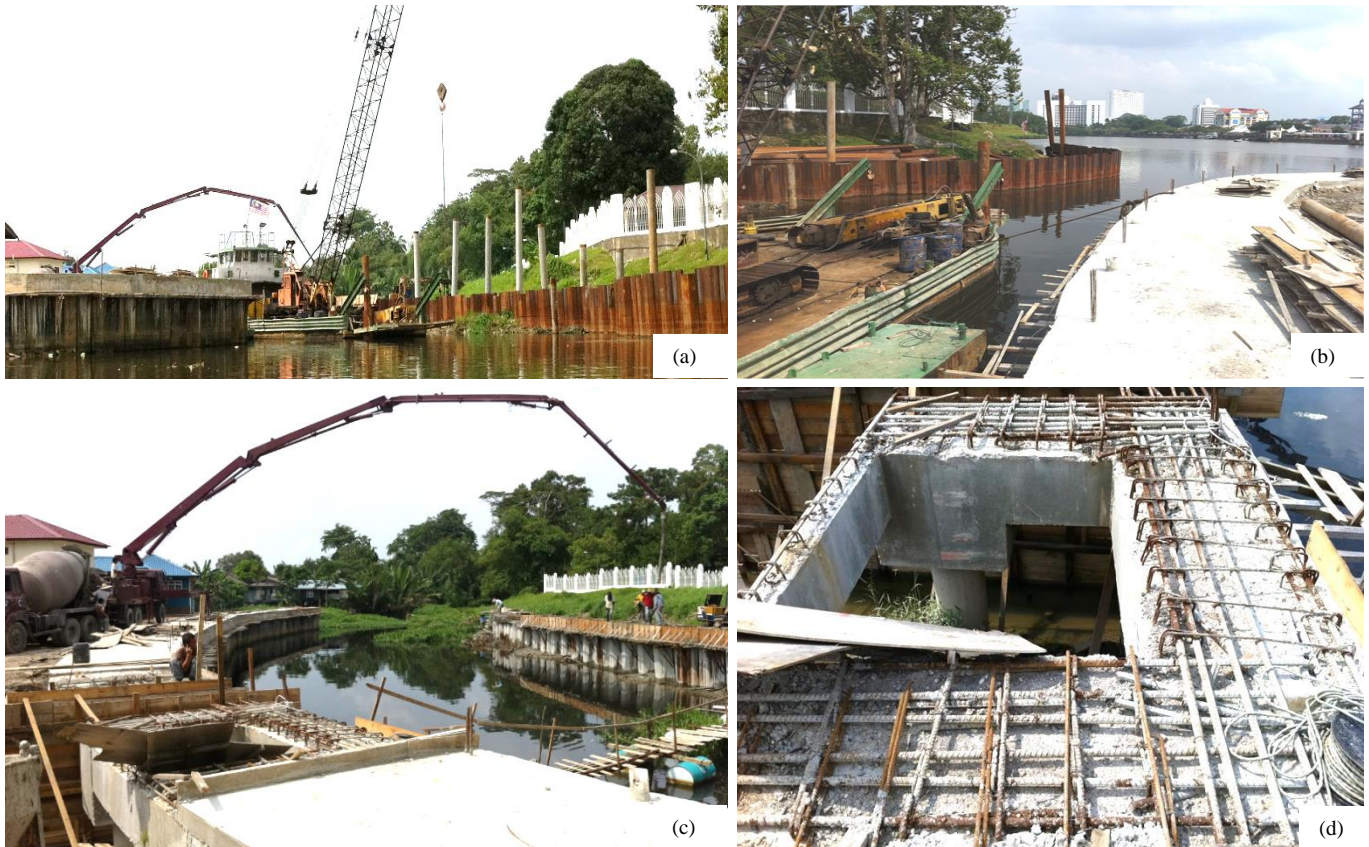
Figure 8. Good construction practices: (a) Use of overhead crane and piling equipment on barge, (b) stable berthing of barge for piling works, (c) use of long-reach concrete pump to relieve unnecessary surcharge load on the soft riverbank and (d) stage-construction of riverwall in progress (Stage 3, note that filling works was intentionally delayed from being placed under the platform until after successful completion of the tie team, which acts as a load transfer mechanism).
