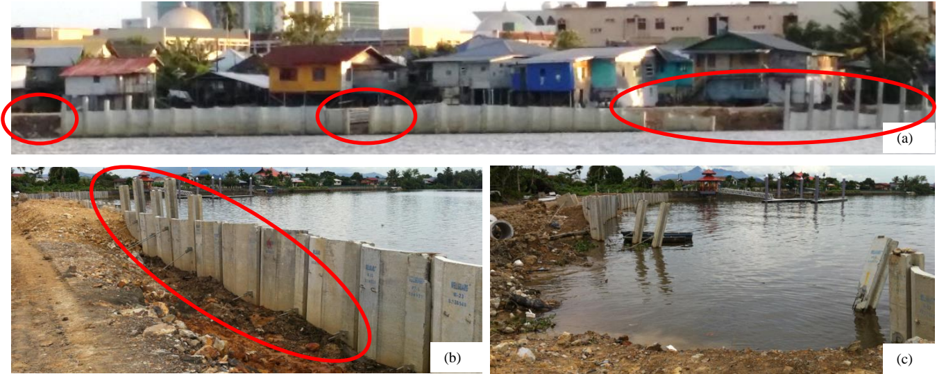
Figure 10. (a) Longitudinal view of 3 locations where circular slips most likely occurred that dragged parts of the concrete sheet pile riverwall system into the river, (b) close-up view showing the haphazard installation of the RC guide piles and anchorage system at grossly different lengths and angles, respectively and (c) close-up view of a major circular slip that might have taken place due to over-loading of the soft riverbank slopes by unplanned filling.
