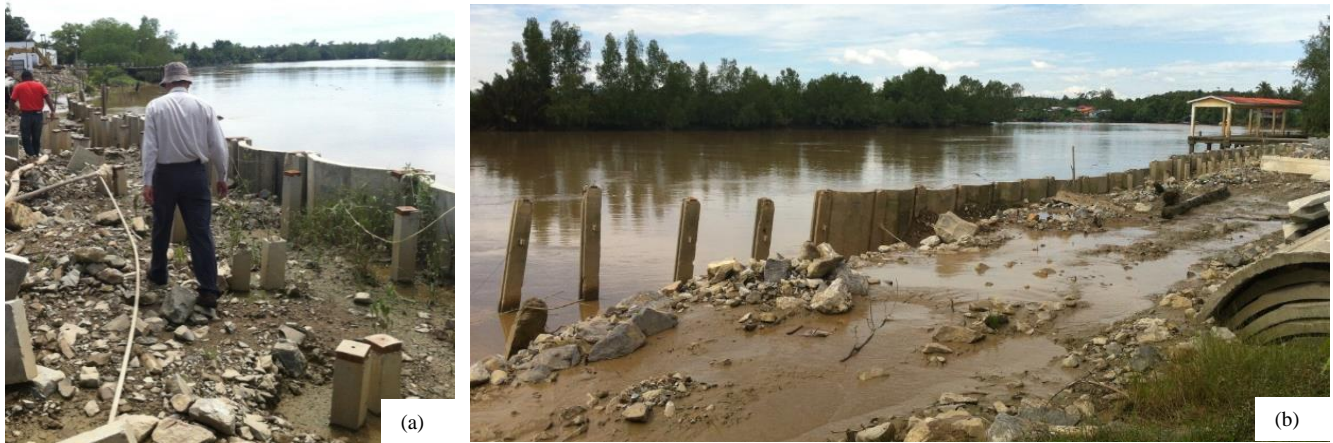
Figure 11. (a) Misaligned concrete sheet pile riverwall system and RC piles and (b) longitudinal view of a major circular slip that might have taken place due to over-loading of the soft riverbank slopes by unplanned filling.
