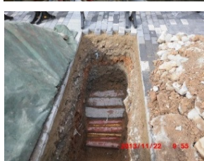
Utilities Congested at Original Working Pit Location
