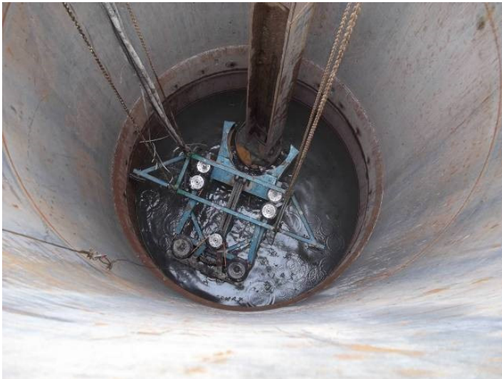
Pile removal by diamond wire saw (courtesy of Victor Li & Associates Ltd)
