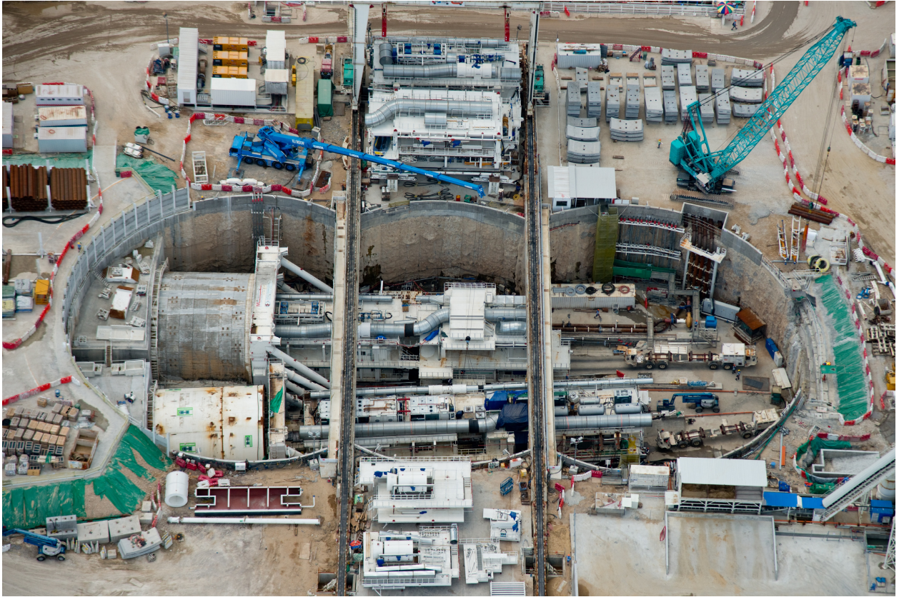
Triple-cell shaft for the Tuen Mun-Chek Lap Kok Link Northern Connection (courtesy of Dragages-Bouygues Joint Venture and Highways Department, HKSAR Government)
