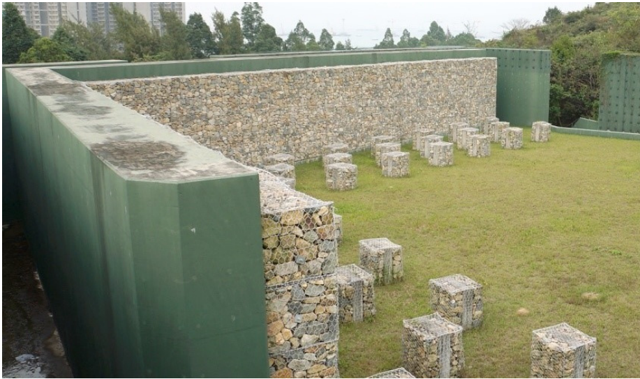
A rigid debris-resisting barrier comprising a reinforced concrete check dam together with gabion cushioning material and baffles (courtesy of Geotechnical Engineering Office, HKSAR Government)
