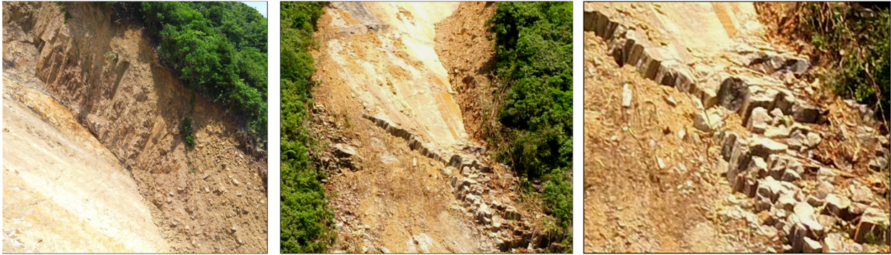
Close-up photos taken by UAV following a landslide above Sai Wan Road in 2016 (courtesy of Geotechnical Engineering Office, HKSAR Government)
