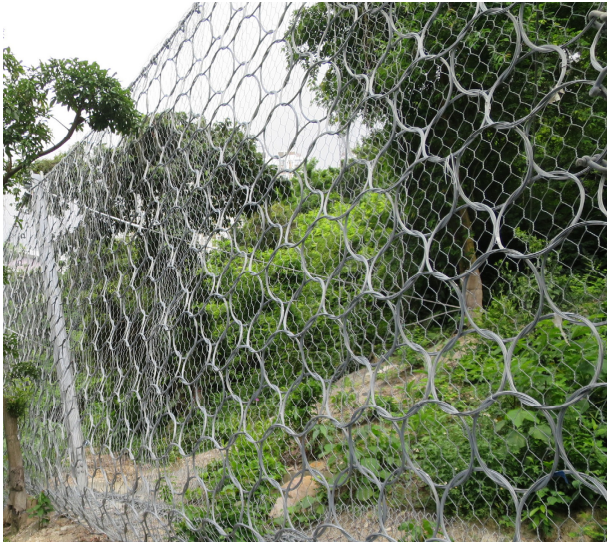
A flexible debris-resisting barrier (courtesy of Geotechnical Engineering Office, HKSAR Government)
