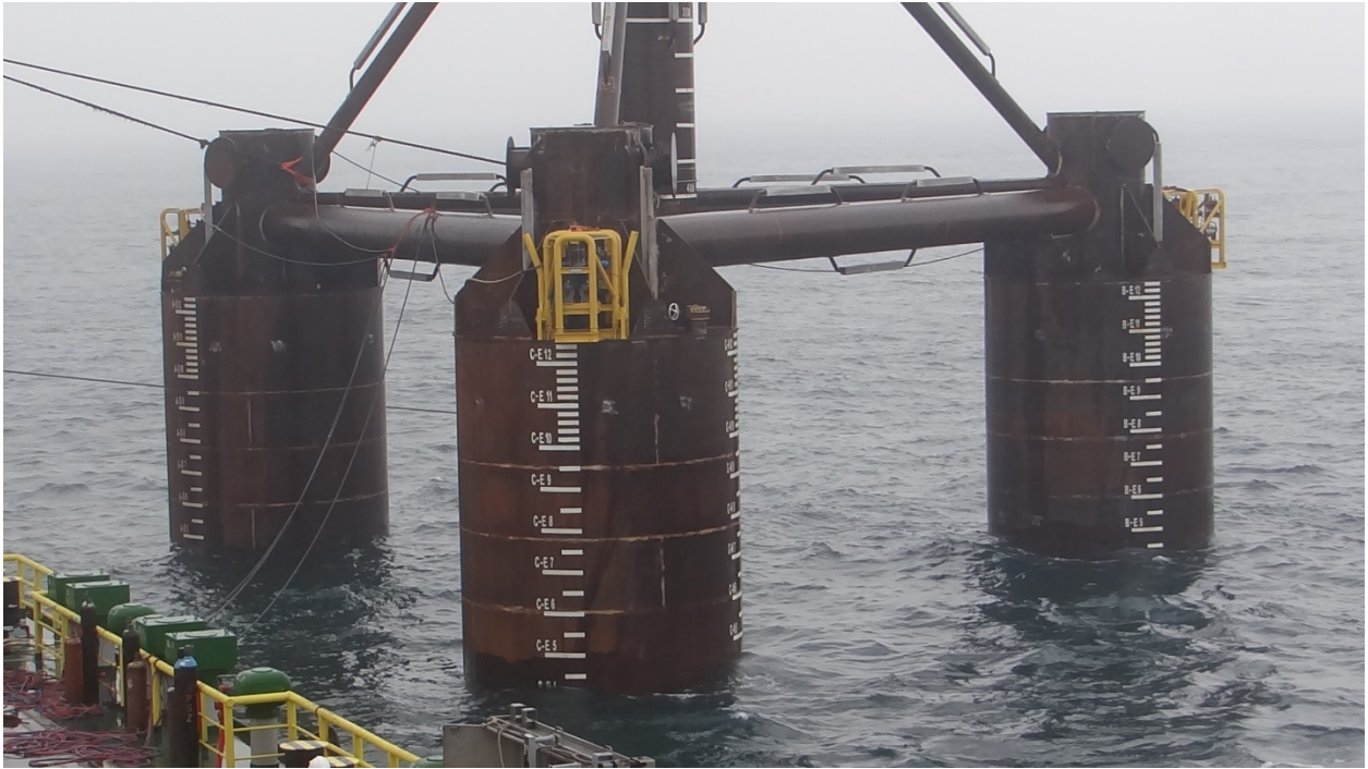
Installation of suction foundation structure (courtesy of Ove Arup & Partners Hong Kong Ltd)
