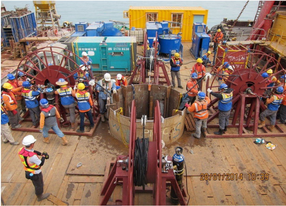
Installation of shaft grouted piles for the Hong Kong-Zhuhai-Macao Bridge (courtesy of Ove Arup & Partners Hong Kong Ltd and Highways Department, HKSAR Government)
