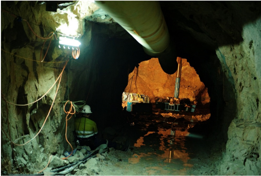
The reamer in position below the pilot hole (courtesy of Dragages Hong Kong Ltd)
