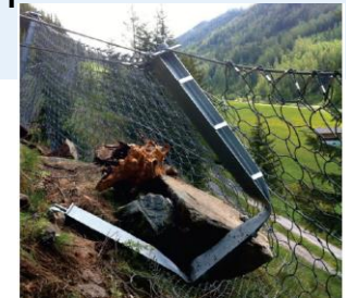
Localised damage of post (Trumer)
