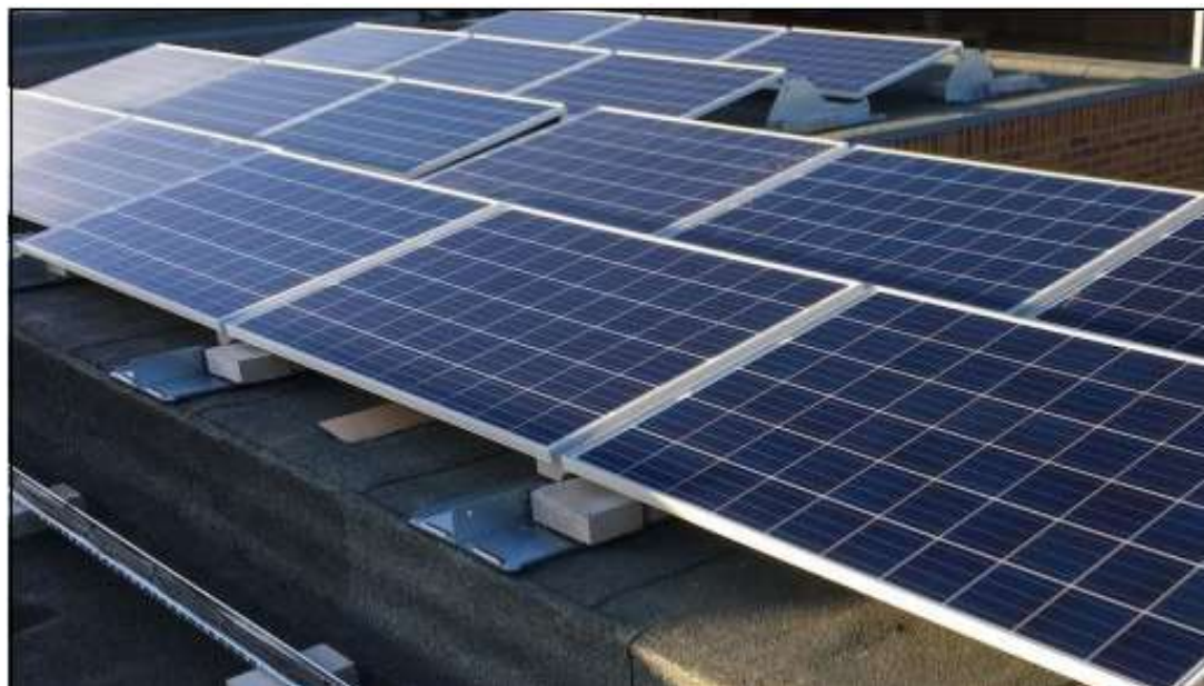
Newly installed solar panels
