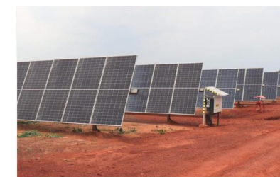
Hybrid & Energy Storage
