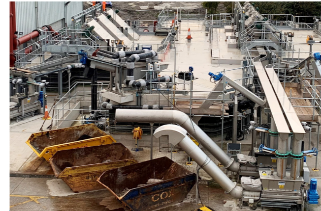
HUBER WAP®L Wash Press installation at Plymouth Central STW serving coarse & fine screens
