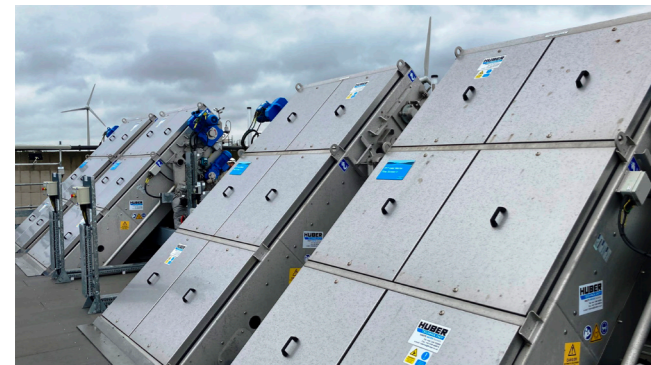
HUBER EscaMax® fine screen installation at Hull WwTW
