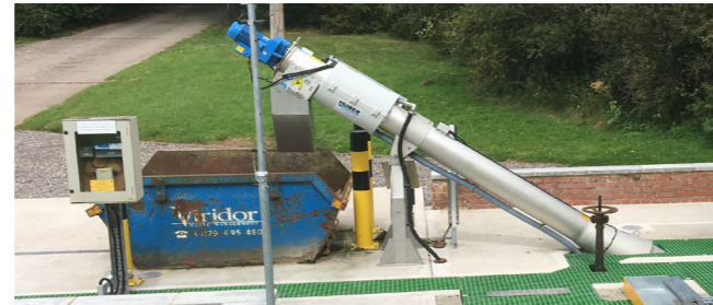
Channel mounted HUBER Ro9 combined screen installation at Michaelwood STW
