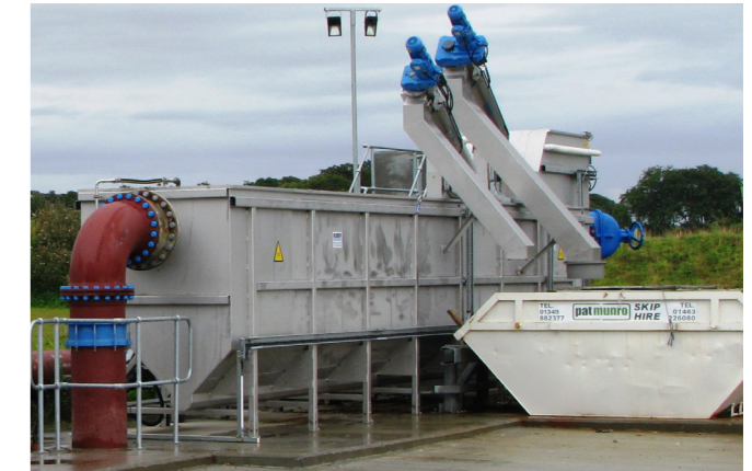
HUBER Ro5 Complete Plant installed at Invergordon STW
