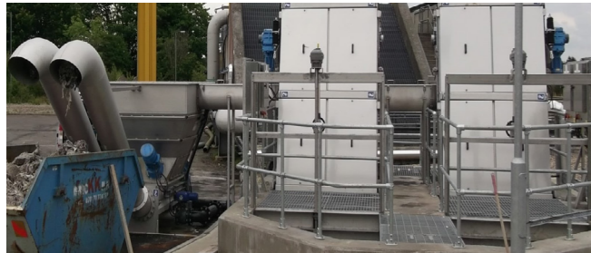
HUBER RakeMax® coarse screen installation at Culmore STW
