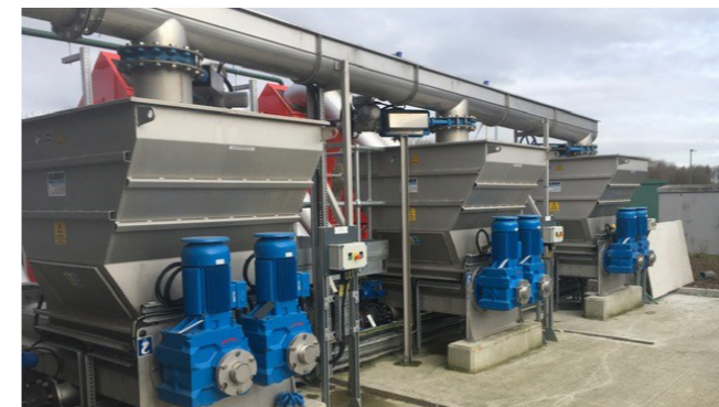
HUBER WAP®SL Wash Press installation at Hull WwTW serving 3 No. HUBER RakeMax® screens
