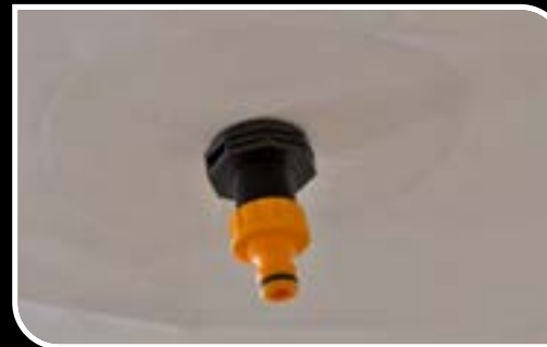
Central Drainage Point
