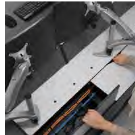
INTEGRATED ACCESSIBLE CABLE MANAGEMENT
