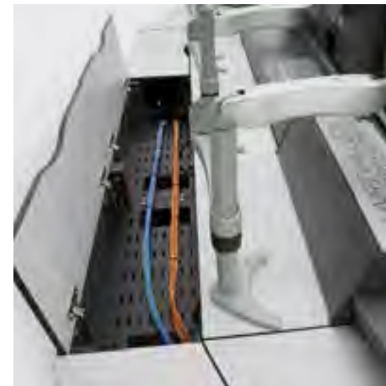
INTEGRATED ACCESSIBLE CABLE MANAGEMENT
