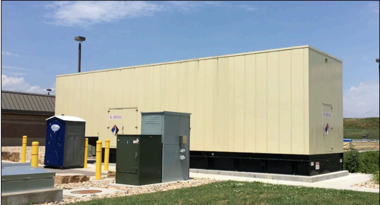
Example Generator Image
