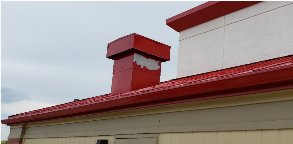
Missing paint identified at the Pizza Hut in Parcel 15736309002
