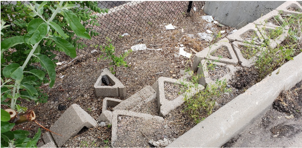
This retaining wall south of the USPS is in disrepair
