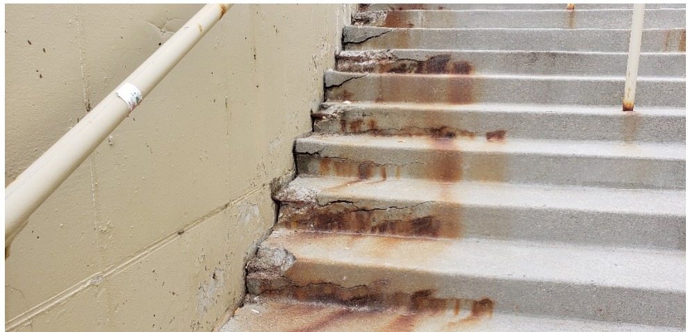
Deteriorating concrete steps observed at the shopping center in Parcel 157536308003
