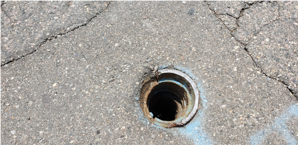
Open, unsecured 6-inch diameter hole (hazard) at Parcel 157536308002
