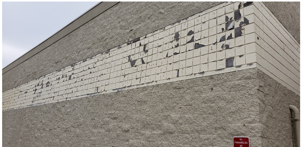
Peeling paint observed on the old Safeway building in Parcel 157536308002
