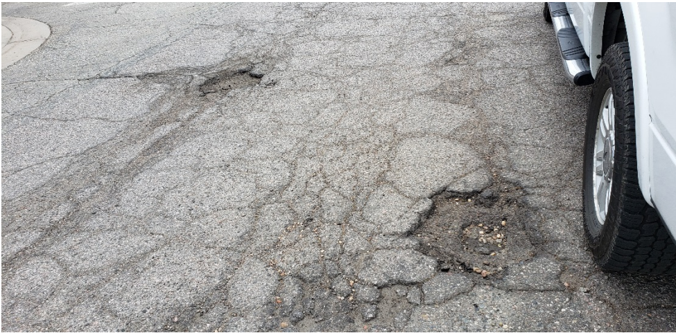
Deteriorating pavement identified in the southern portion of the Study Area
