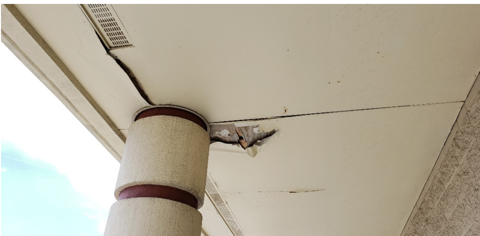
Deteriorating wood fascia identified at the former Safeway, Parcel 157536308002
