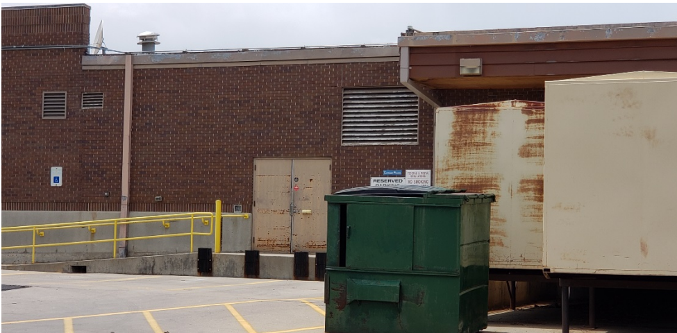
Rusting metal doors and storage container observed at the USPS (Parcel 157536302002)
