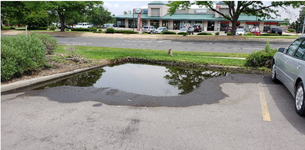
Inadequate drainage, standing water at Parcel 157536309004
