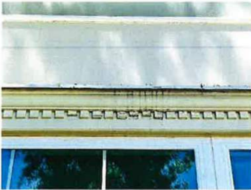
11. Damaged wood trim east bay window
