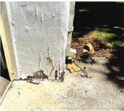
13. Peeling paint on northeast side of home
