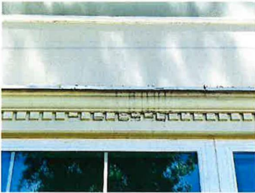
11. Damaged wood trim east bay window
