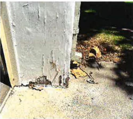
13. Peeling paint on northeast side of home
