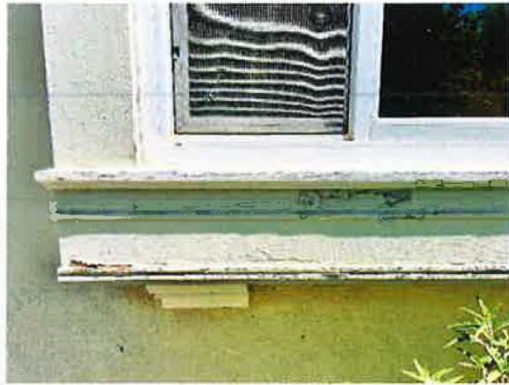
12. Peeling paint, damaged wood trim south bay window
