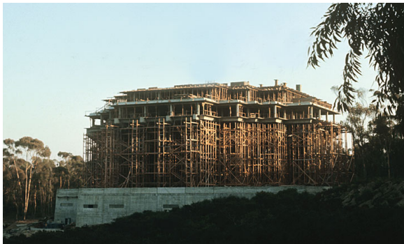
Geisel Library under construction in late 1969. From "Celebrating the University's Built Environment" in UC San Diego Annual Financial Report 2009–2010.
