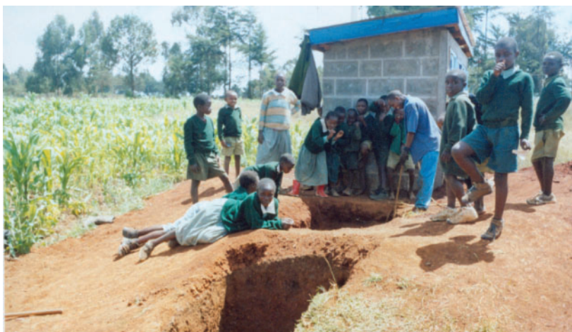
Figure 3 Latrines, like these under construction at Madaraka Public School, Kenya, provide students with a safe, private, and dignified place to eliminate bodily wastes.
