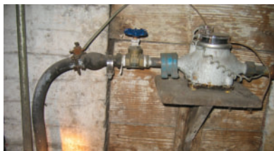
Figure 1 Water pipes or connectors made of lead can be a source of lead contamination in the drinking water of older homes. The pipes connect the home plumbing system to the public water main under the street.
