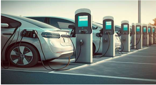
EV Charging Stations
